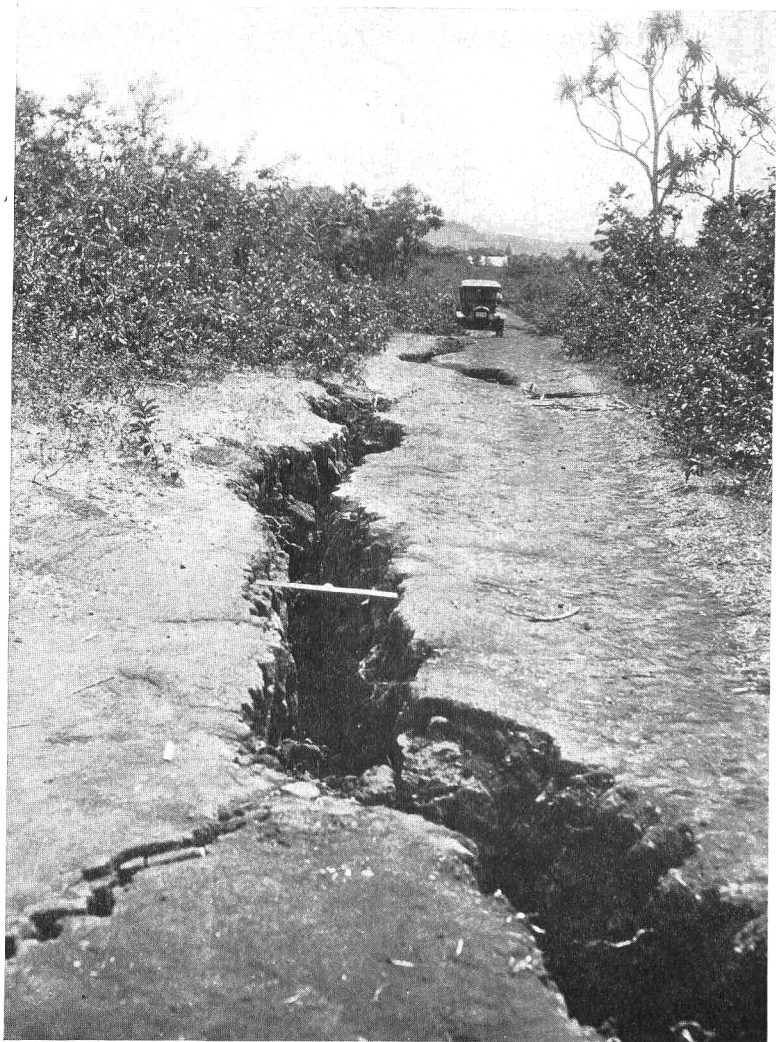
FIG. 2.—Cracks two feet wide, looking southwest toward Kapoho village. About April 24, 1924. Photo by Tai Sing Loo.
